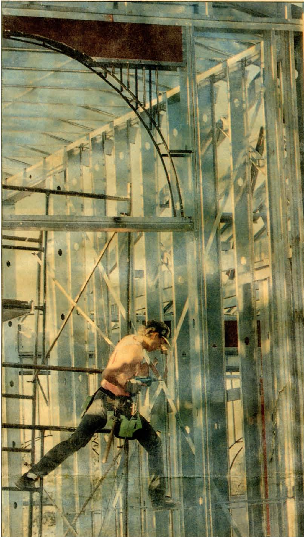
R-S photos by Rollin Banderob Dan Caton of Redding uses a screwdriver this week to attach diagonal bracing strips at the entryway to a steel-framed house under construction in Palo Cedro.
